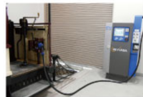
急速充電風景 Rapid charging
