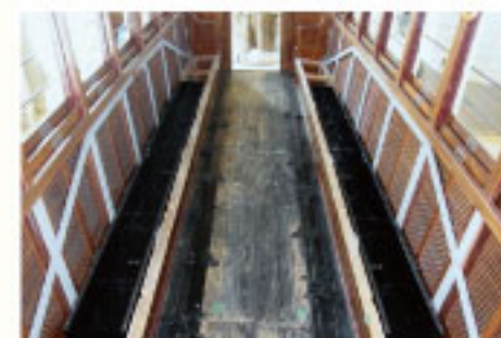
座席下バッテリー収納 Under-seat battery installation
